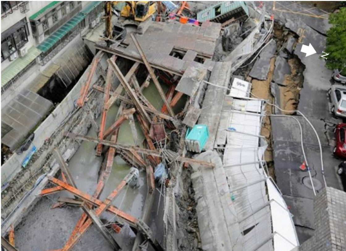
Figure 8. Collapsed slurry wall retaining structure of the Jitai-Dazhi site during the foundation excavation.
