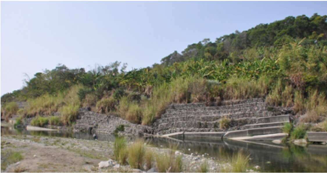
Figure 2. Piping failure of the gabion retaining wall (Toubiankeng Creek in Taichung, Taiwan).
