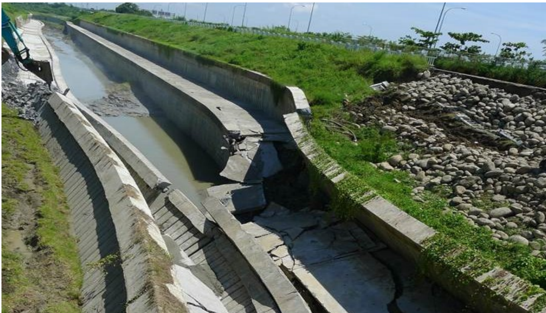
Figure 3. Piping failure of the retaining walls on both sides of the floodway (Gangweigou Creek in Tainan, Taiwan).
