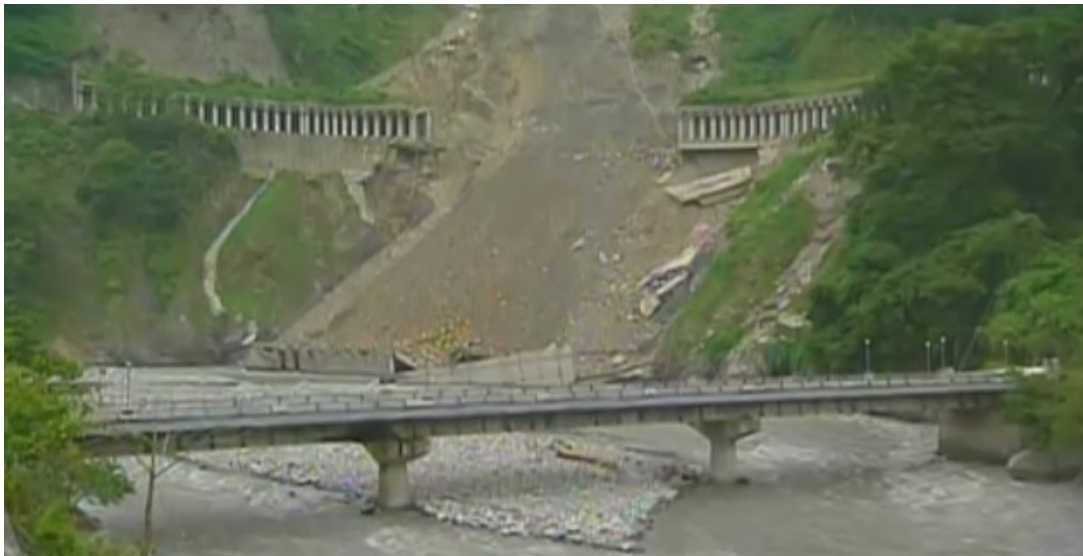
Figure 1. Piping failure of the retaining wall of the open-cut tunnel (Central Cross Highway in Taichung, Taiwan).
