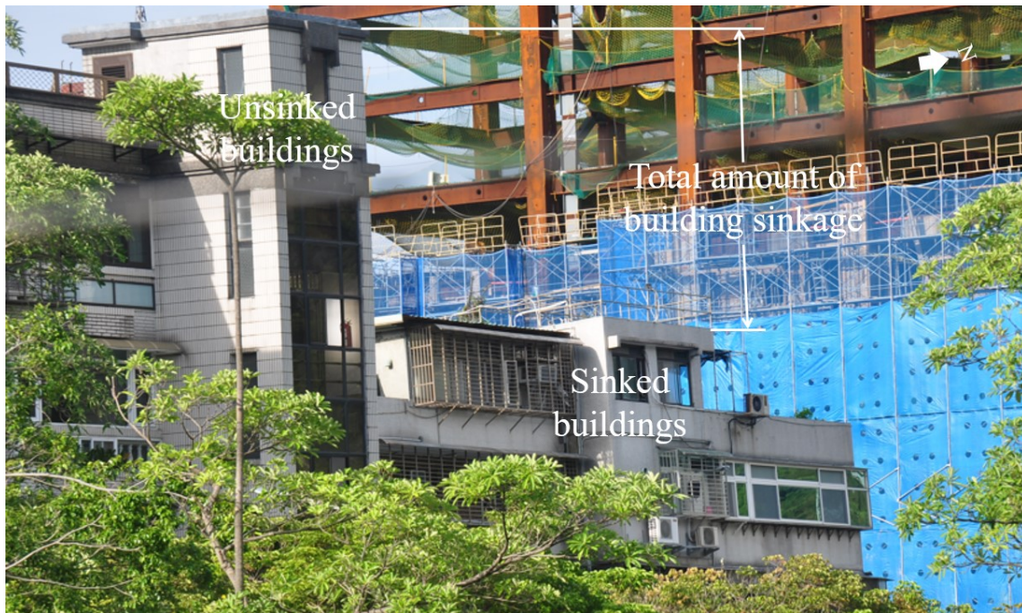
Figure 9. Subsidence of the building adjacent to the Jitai-Dazhi site during the foundation excavation.
